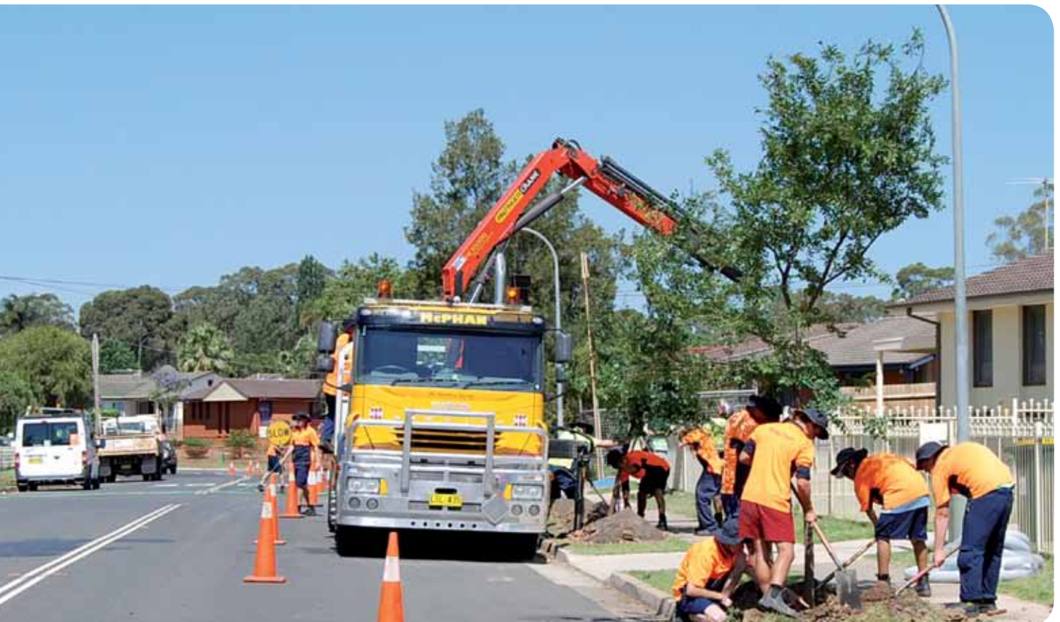
The pilot crew planting 200 litre, 3.5 metre high trees in Chestnut Crescent, Bidwill, NSW.
